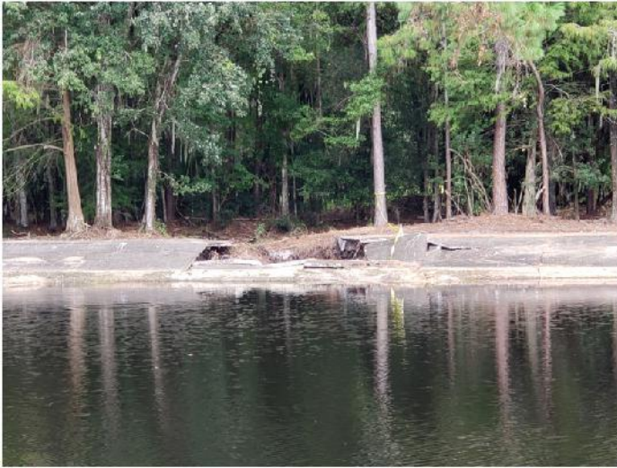
Weir wall section collapsed
